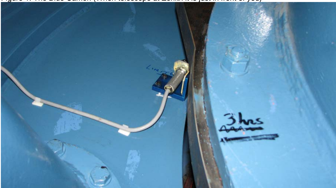
Figure 2: The East Below Pole Limit Switch. (When telescope at Zenith it is at your left side)
